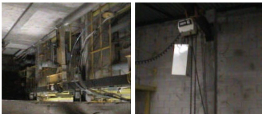
Figure 2. Elevator shaft area and the 3-ton crane for the drop box experiments
